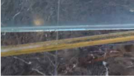
Case in Point 3: Shower door seal (broken and unclean)
